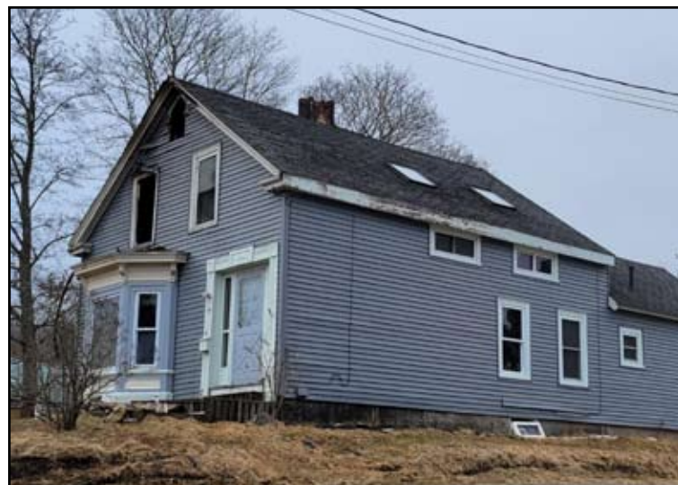
A fire that likely began in a chimney spread to this School Street home's attic last week. Photo by Sarah Craighead Dedmon
