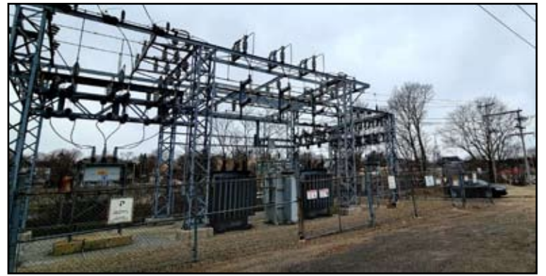
Long-standing plans to relocate this less-than-scenic electrical substation away from scenic Bad Little Falls Park are still in the works, according to Versant spokesperson Judy Long. Machias Town Manager Bill Kitchen said the town is not looking to sell one of its tax-acquired properties in case it suits as an alternative site for the substation. Photo by Sarah Craighead Dedmon
