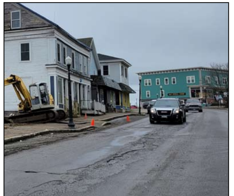
A rutted Route 1 through Machias is seen earlier this year before Maine DOT performed maintenance shim work to fill the potholes. Now, Maine DOT will receive $33M in federal INFRA funding to rehab almost 70 miles of Route 1 between Machias and Calais. Photo by Sarah Craighead Dedmon
